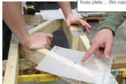
Photo no. 126 Truss on site ready for installation. Gap between truss plate... (No capacity beyond 3/32" gap).
